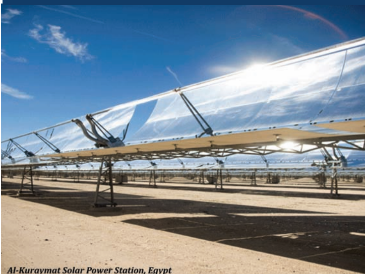
Al-Kuraymat Solar Power Station, Egypt
